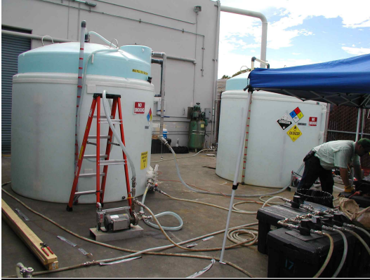
FIGURE 3. Hydrogen peroxide tanks used for activation of persulfate.
