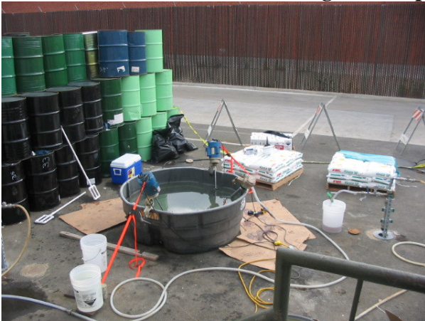
FIGURE 1. Tank used for mixing sodium persulfate
